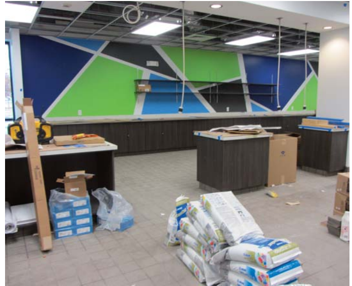
Work on the new Meals on Wheels kitchen and office area is nearing completion.
